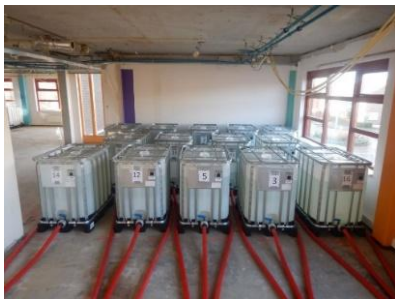
Fig. 8a. Proof loading of a floor of an office in Leidschendam, Netherlands.
