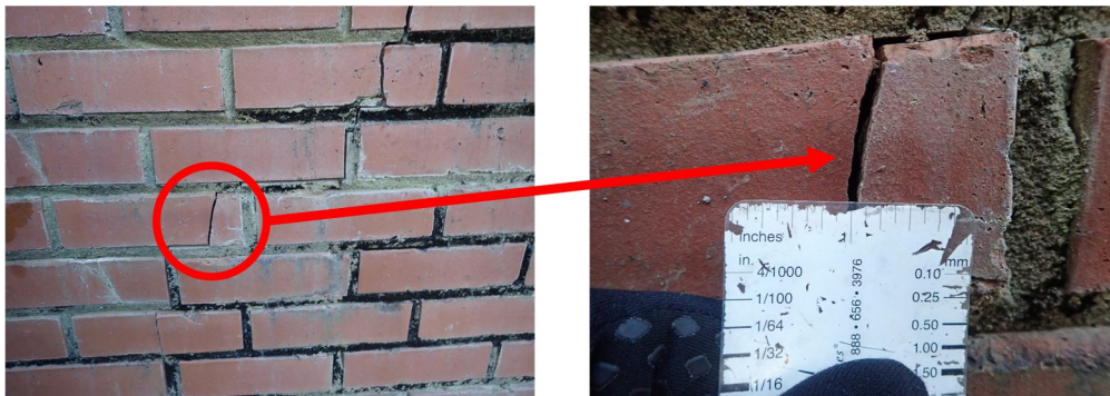
Figure 6. Cracking in a brick wall. Note the rounded edges of the crack indicating it did not form recently.
