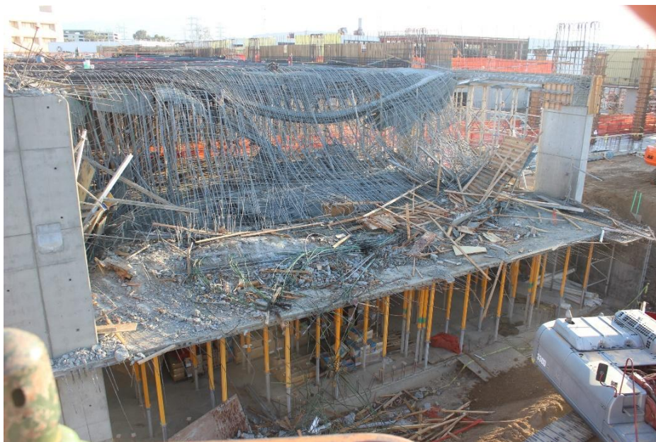
Figure 5. Partial collapse of a concrete structure during construction.
