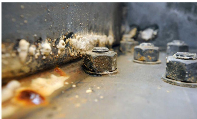
Figure 1. Evidence of corrosion around bolts in the San Francisco-Oakland Bay Bridge (photograph courtesy of SF Chronicle).
