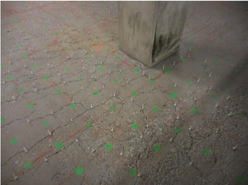
Figure 4. Cracking in an elevated, two-way concrete slab, which is prepared for repair using epoxy injection ports.
