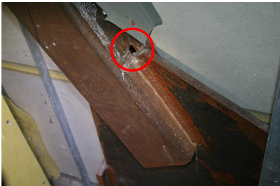
Figure 7. SCBF diagonal-to-gusset plate connection with a hole left in the connection (indicated).
